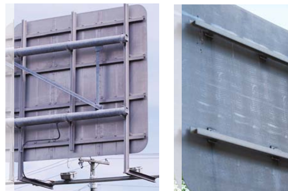
Aluminum Z-bar on an overhead guide sign
